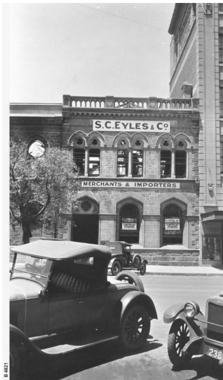
State Library of South Australia - Currie Street, Adelaide [B 4821], [General description] S.C.Eyles' building is in process of demolition with street and parked cars in the foreground. [On back of photograph] 'Acre 136 / Currie Street, south side / 10 January 1928 / Eyles' premises demolished in 1928. For view of building erected in 1929 see B 5430 / Site of Eyles' premises: Left side is 19 yards west of Bloor Court / Frontage: 10 yards'. Approximately 1928. Photographer, State Library of South Australia. Part of Acre 136 Collection.
